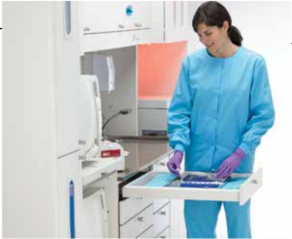
Contained under the single countertop, the nurse is able to wrap the cassette for sterilisation.
